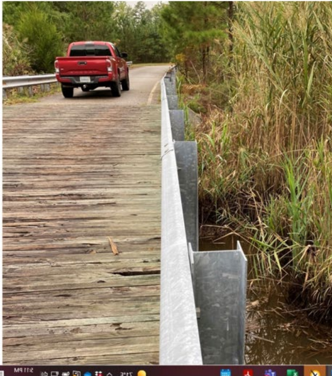
Image 1- Failing decking due to rising flood waters
