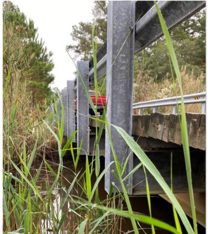
Image 2- Elevation is less than two feet above flood level
